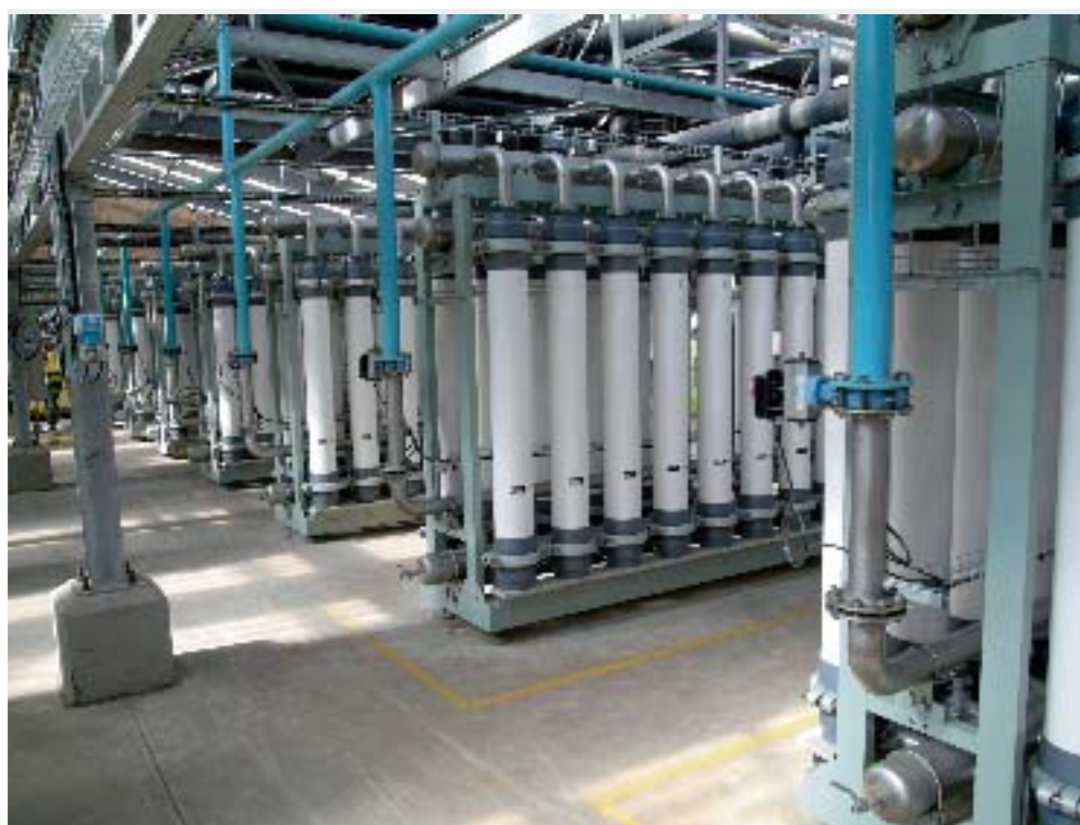
Reverse Osmosis plant in South Africa used to transform coalmine waste water into water fit for the municipal supply
