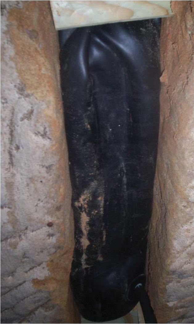
Figure 6: The fissure is 150mm wide at this point
